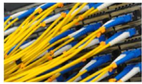
Fibre Optic & Data Structured Cabling System
